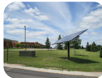
Photo: Solar Energy System, River Falls High School, Pierce Co., WI.
