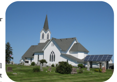
Photo: Solar Energy System, Town of Ellsworth, Pierce Co., WI. Our Saviors Lutheran Church.
