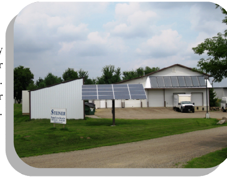
Photo: Solar Energy System, City of River Falls, Pierce Co., WI. Paul Steiner, Steiner Electric.
